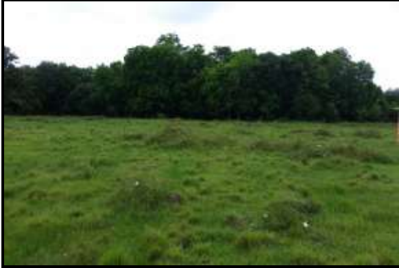
View looking east at the temporary construction area near the northern project limits.
