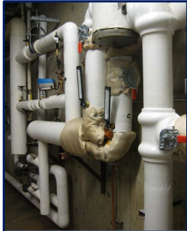
AHU-1/2 combined steam to hot water converter
