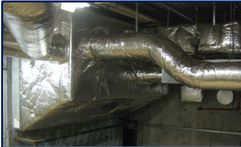
AHU-1 Supply Air Plenum
