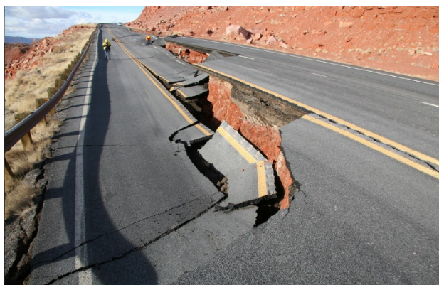
Photo of Collapsed Section of U.S. Route 89
