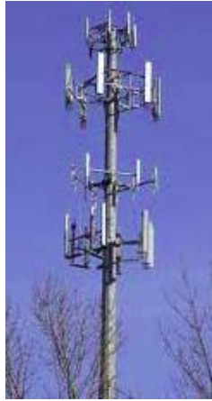
Figure 2.4.3-1: Monopole Cell Tower with Multiple Panel Antennas
