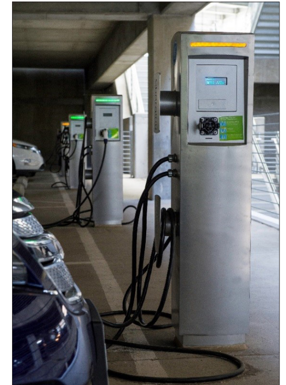
Electric Vehicle Charging Stations. Image source: Alternative Fuels Data Center (AFDC)
