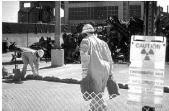
Hazard area secured with fencing and signs
