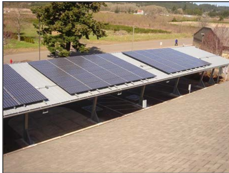
42-kW PV panels installed on Grand Ronde Tribal Housing Authority carport. Combination of tribal funds and state incentives. Photo from GRTHA, NREL 31797
