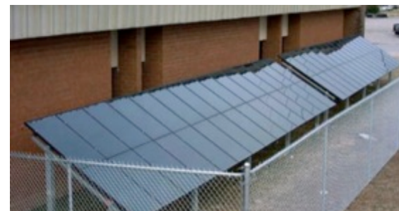
NC Solar Center, NREL 09373
