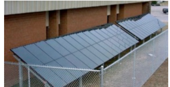
NC Solar Center, NREL 09373
