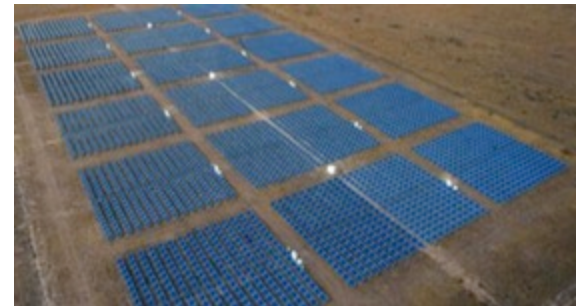
Tucson Electric Power, NREL 13327
