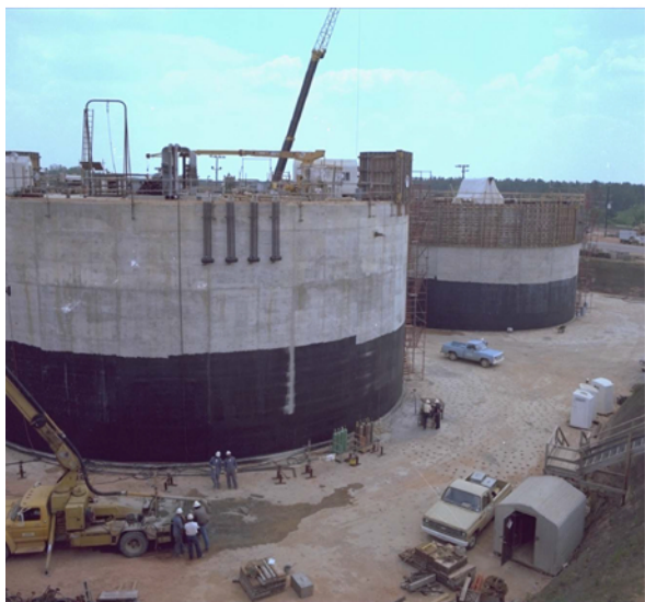
High-level Waste Tank
