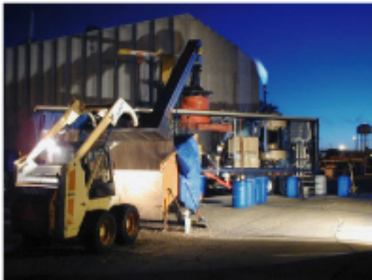
Example of feeding during the first night of operation
