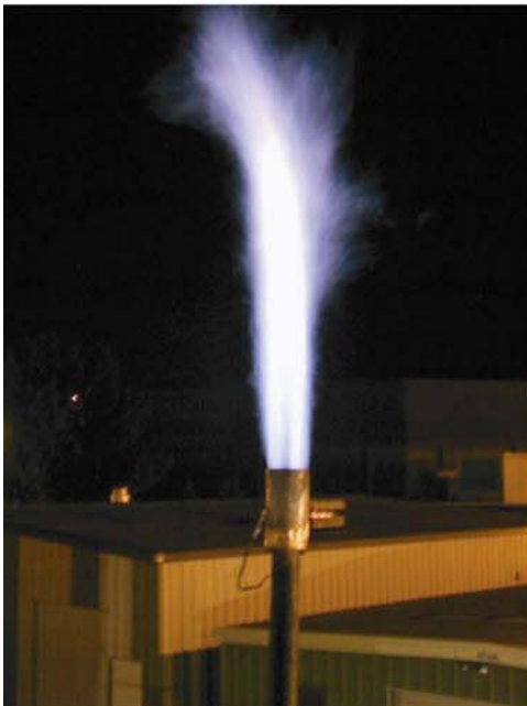
Flare – Product Gas – Nighttime operation
