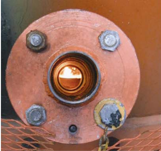
Looking into the Air Nozzle (combustion zone) Inside the Gasifier
