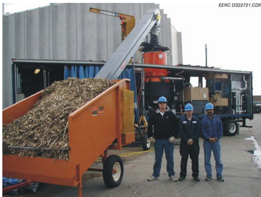
Figure 2. The EERC's portable 150-kW power system.
