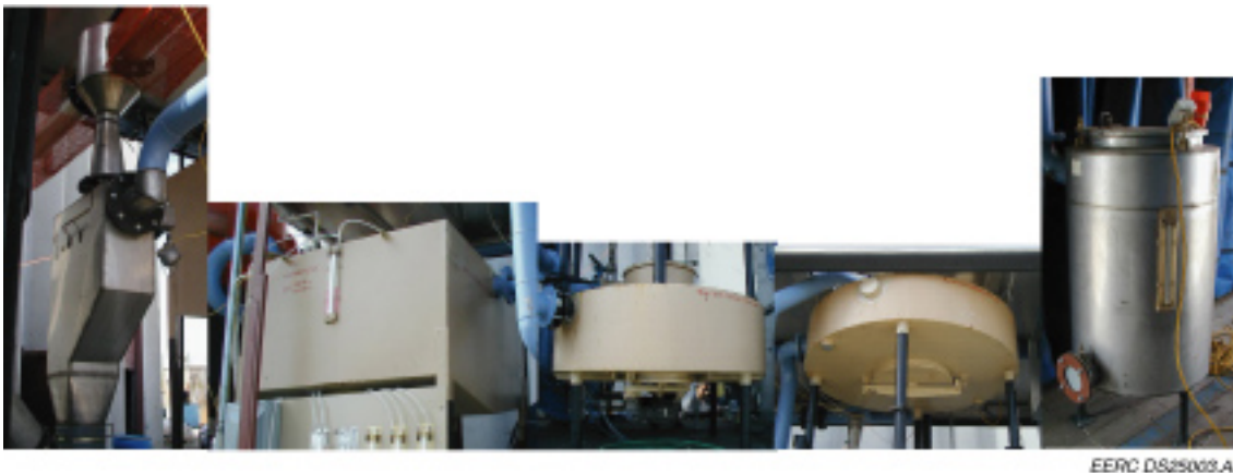
Figure 6. Venturi scrubber and filtration system – from left to right: scrubber, coarse filter, fine filter active, fine filter passive, and safety filter.
