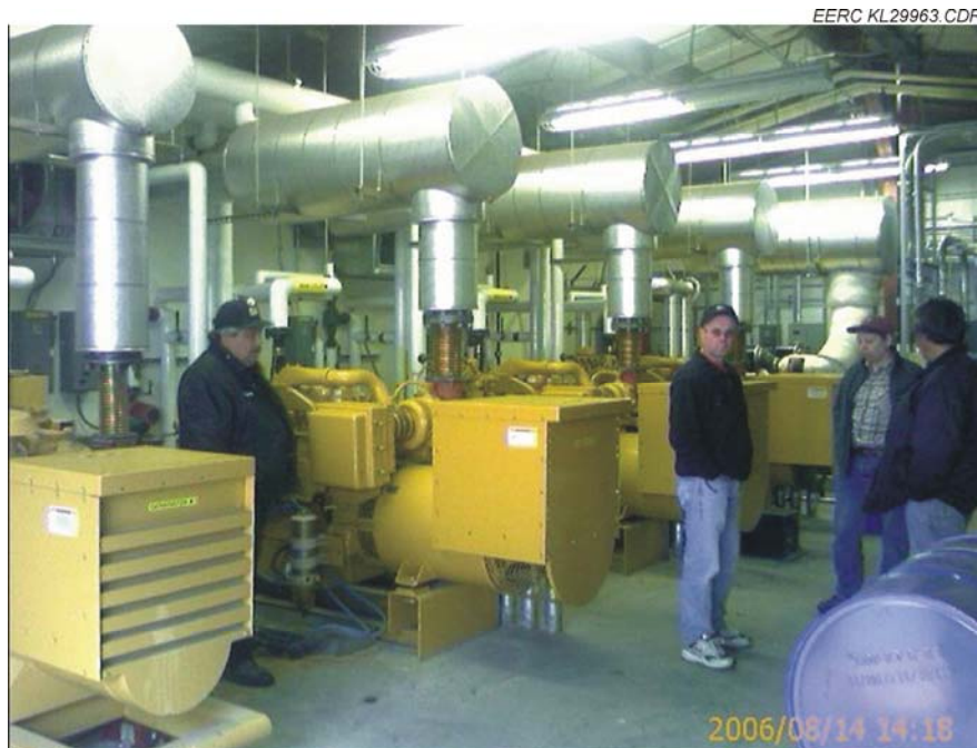
Figure 3. Port Graham Power Plant.
