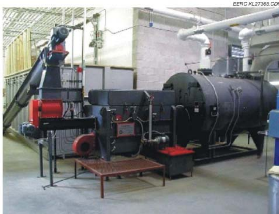
Figure D-7. Chiptec gasifiers and boiler system (Chiptec Wood Energy Systems, 2006).
