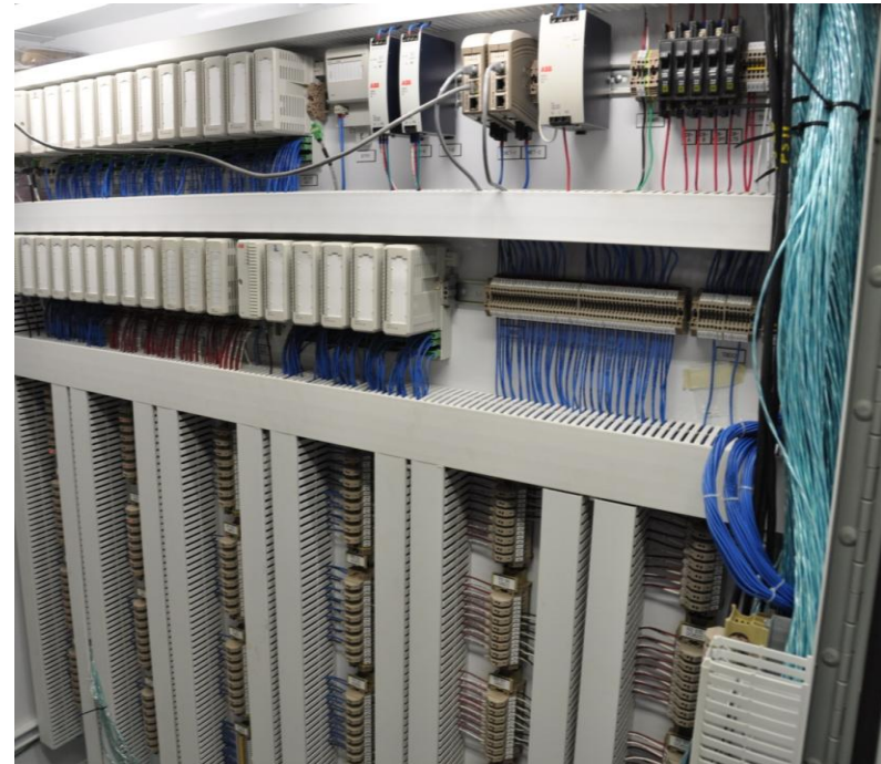
Figure 3. IO panel for the process instrumentation and control.
