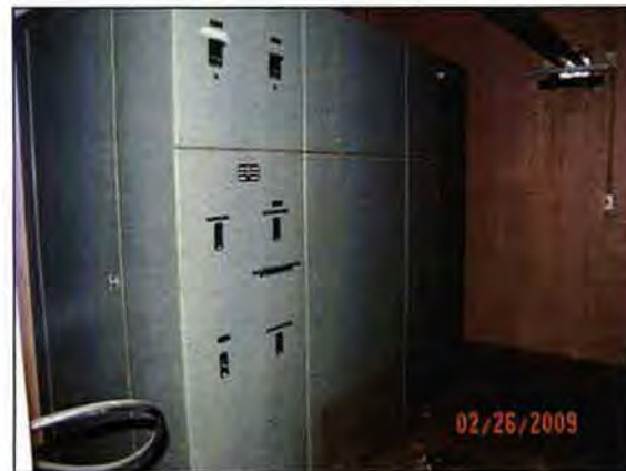
Electrical load center
