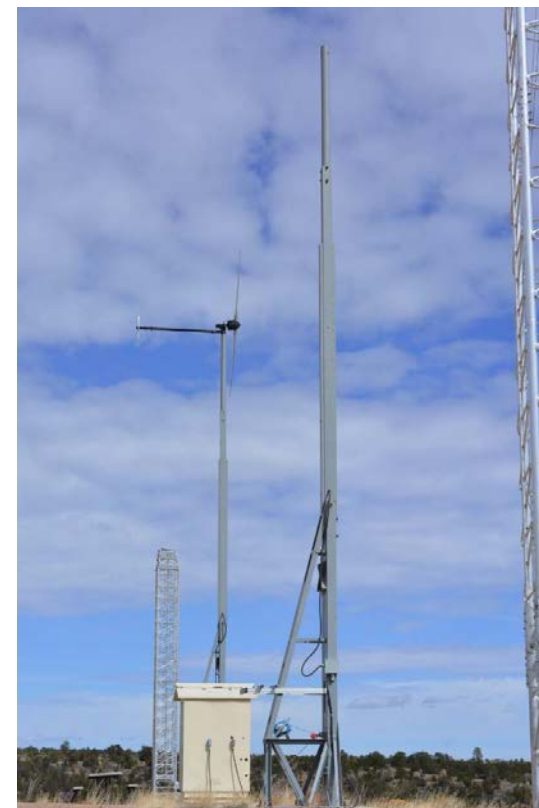
Coupled Wind Turbines
