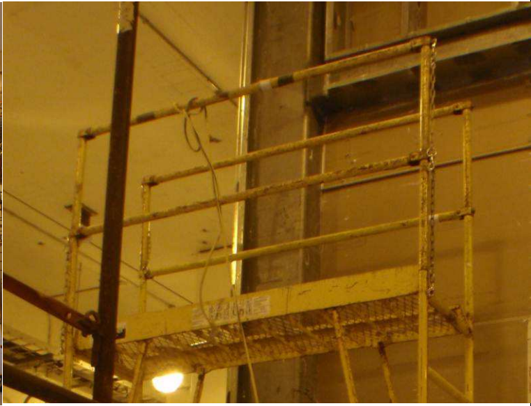
Figure 2-22: Tele-Tower@ A Safety Chains unhooked
