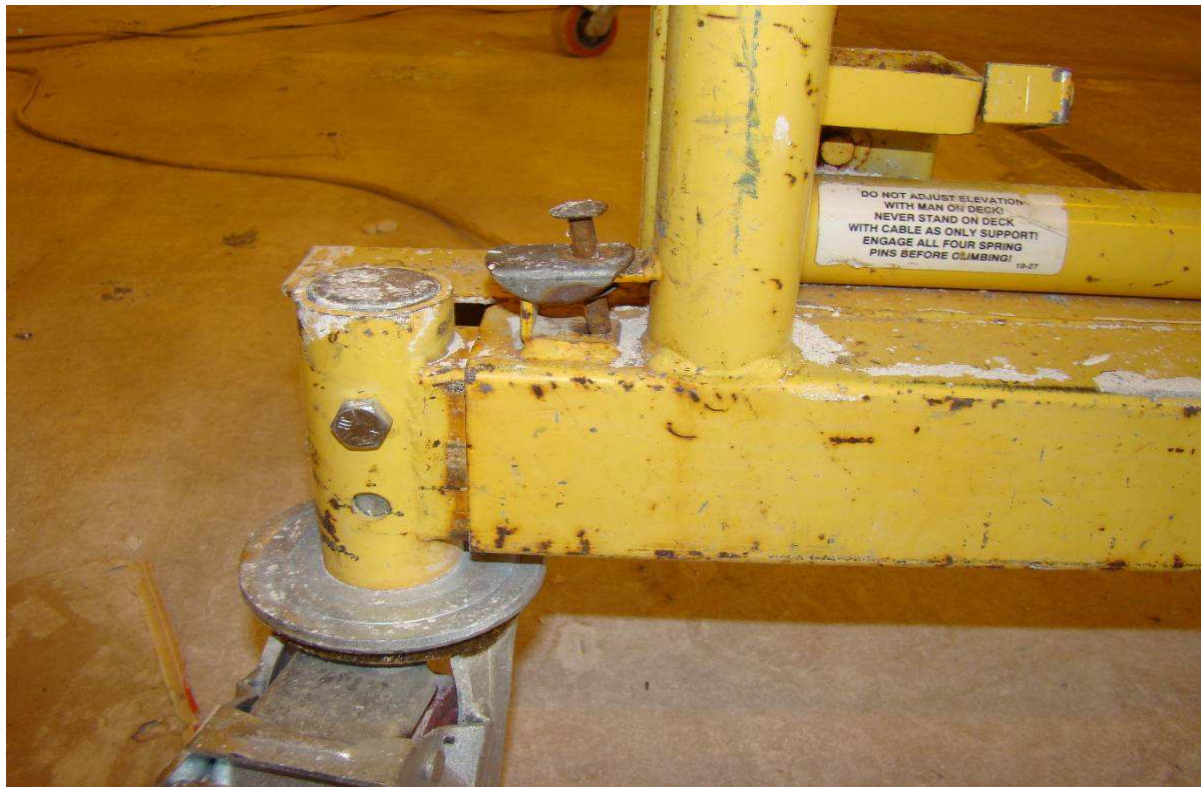
Figure 2-66: Example of locking pin not properly engaged on Tele-Tower® B
