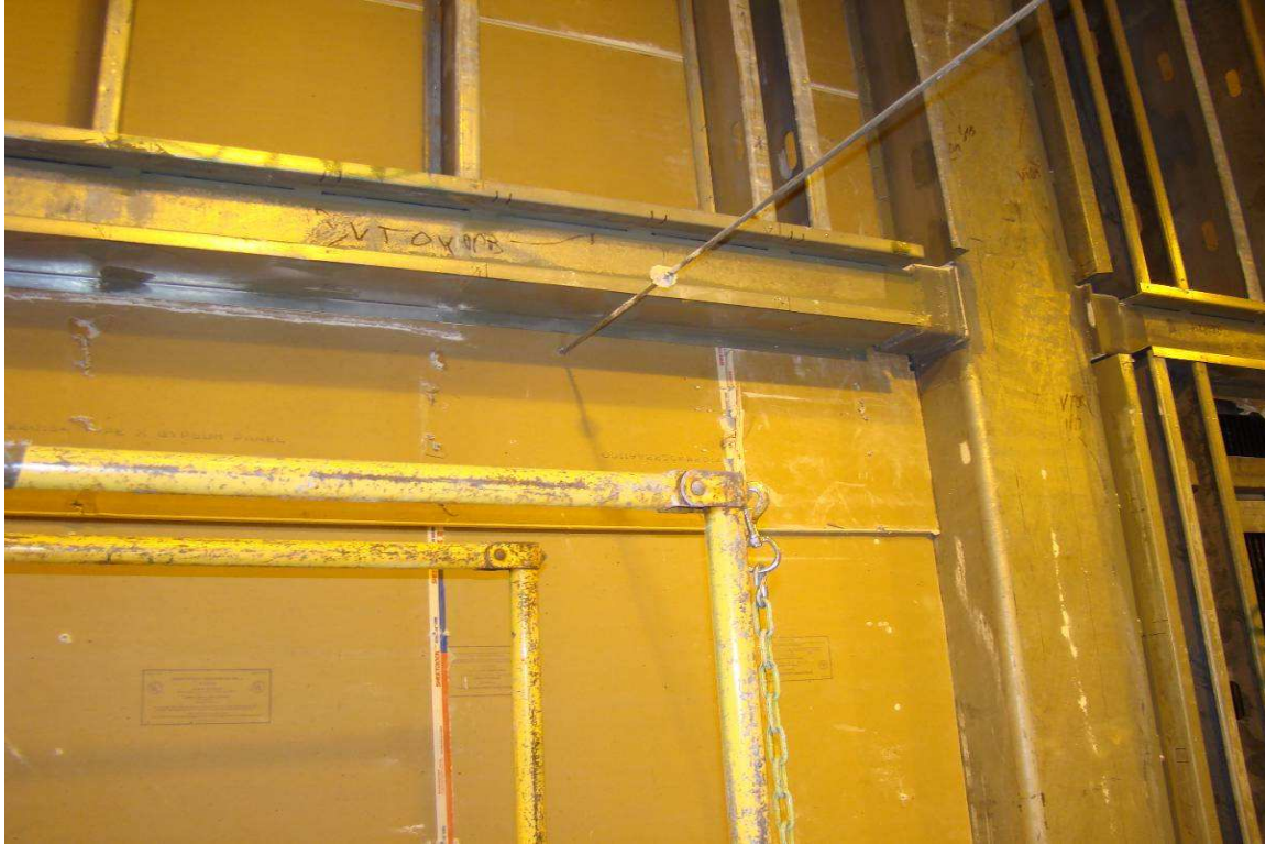
Figure 2-77: Cable near end of scaffold where IW fell
