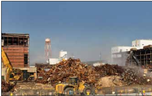
Workers have taken out a middle piece of K-25’s east wing to isolate the technetium-contaminated south end. Demolition of the north end of the wing can now proceed.
