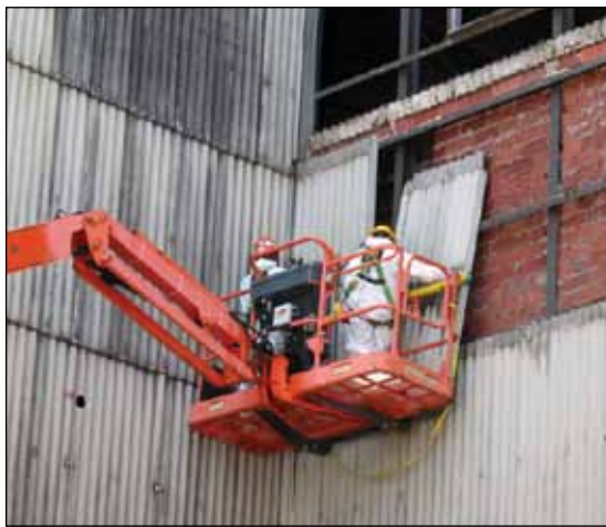
Workers began removing the transite panels from the last section of the K-25 Building in late May. Final demolition will begin this fall.
