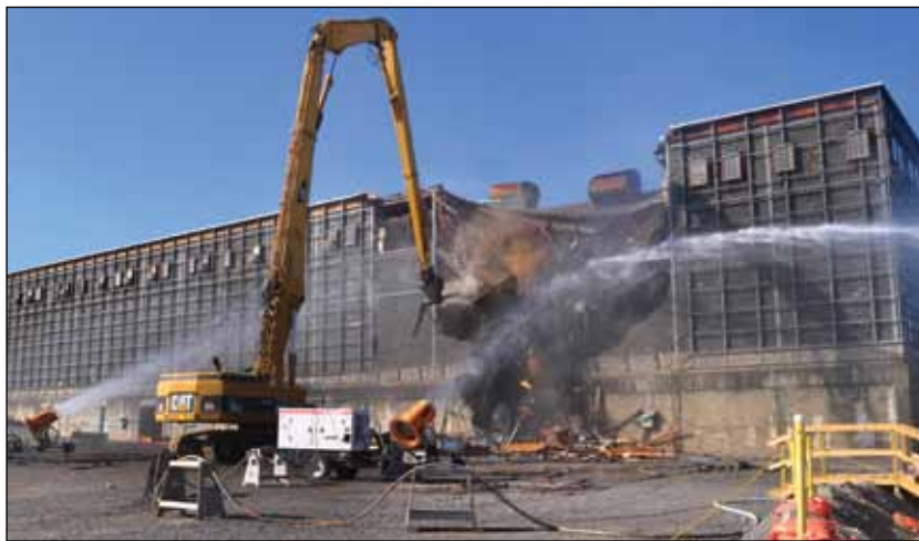
Demolition of the North Tower of the K-25 Building at ETTP began October 23.
