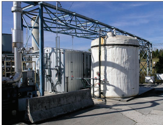
The new Chromium Water Treatment System at ETTP converts chromium-6, which enters Mitchell Branch through groundwater, into chromium-3, a safer form of the element.
