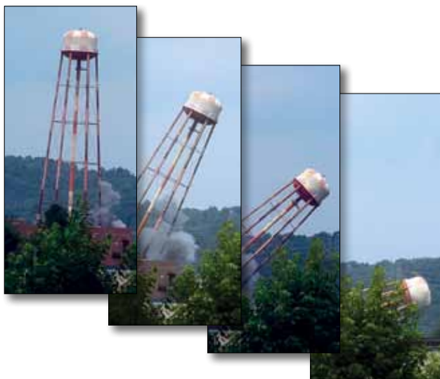
Going, going, going, gone! The iconic water tower at ETTP comes tumbling down after a controlled demolition in August.
