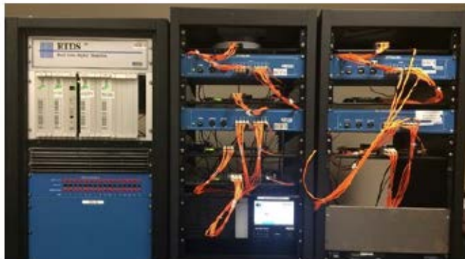
RTDS and MMC support unit hardware
