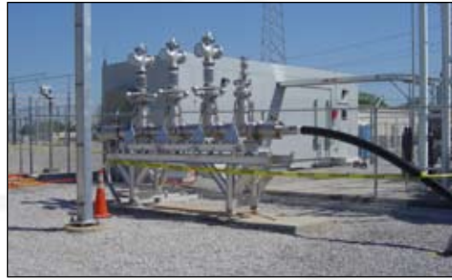
13 kV Triax cable terminations fully assembled at AEP's Bixby station.
