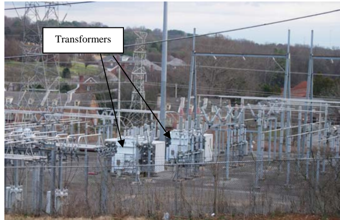
Fig. 4. A utility substation with both modern transformers and bus structure.
