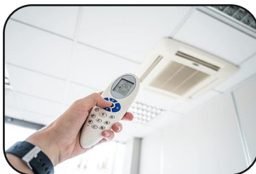
Guidance on Control Systems
