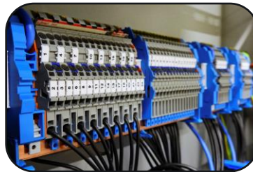
Preliminary Electrical Panel Assessment
