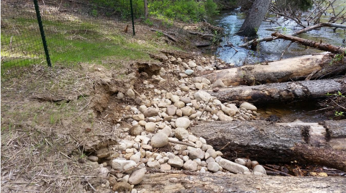
Figure 57: Example of previous in-stream wood placement along the Chewuch River. The bare soil was seeded and the riparian planting were on the other side of the mesh fencing. Rock armoring along the stream bank would help reduce erosion.
