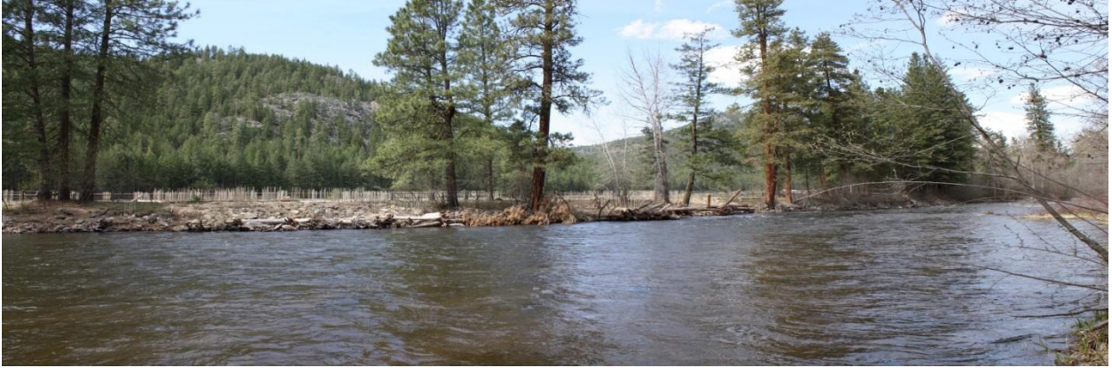
Figure 40. Photograph looking upstream at the constructed log structures on the south end of Eightmile Ranch riverfront.
