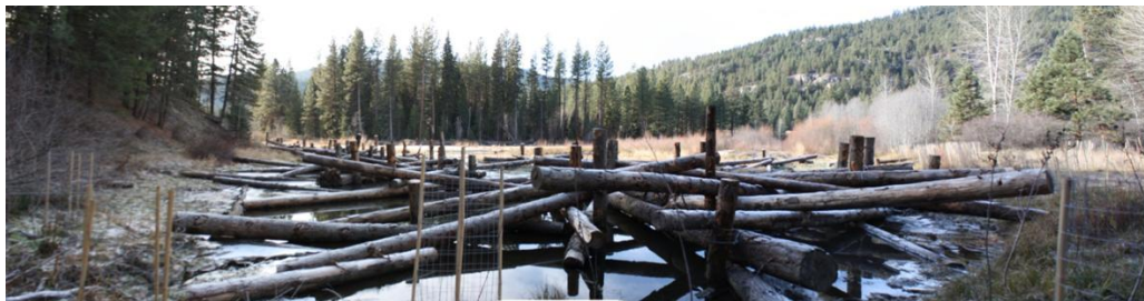
Figure 43: View of Structure 13B from the user-created trail leading to the backwater area.
