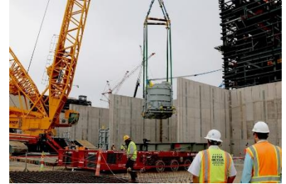
Vogtle 4 step-up transformer is lifted into place. (Courtesy of Georgia Power/ Southern Company, May 2018)
