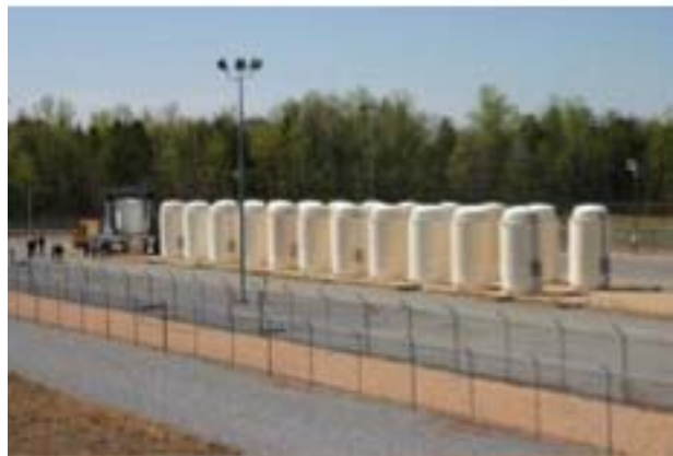
Figure 3-1: Placing Dry Storage Casks on the ISFSI Concrete Pad at North Anna.
