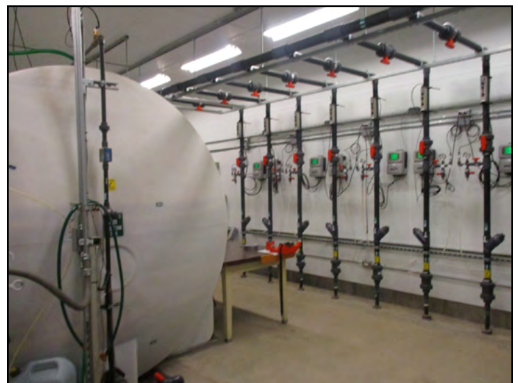
Interior of groundwater transfer building.
