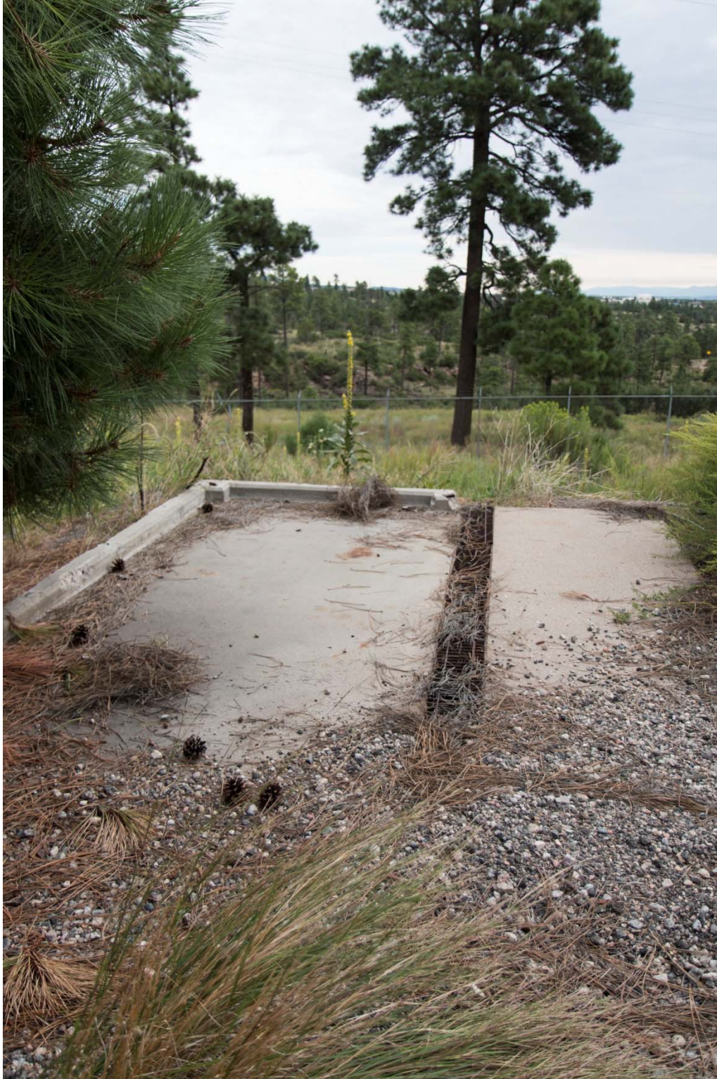
Figure I-13 Trench drain connected to eastern outfall at AOC 15-014(h) with asphalt debris, looking northeast
