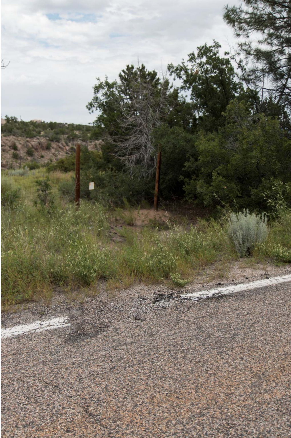
Figure I-18 Weathered asphalt at Potrillo Drive draining to SWMU 36-003(a) drain field, looking north
