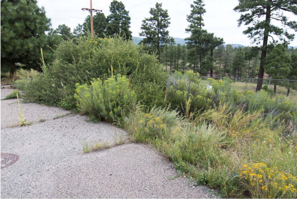
Figure I-14 Weathered asphalt pad above AOC 15-014(h) outfalls, looking northeast
