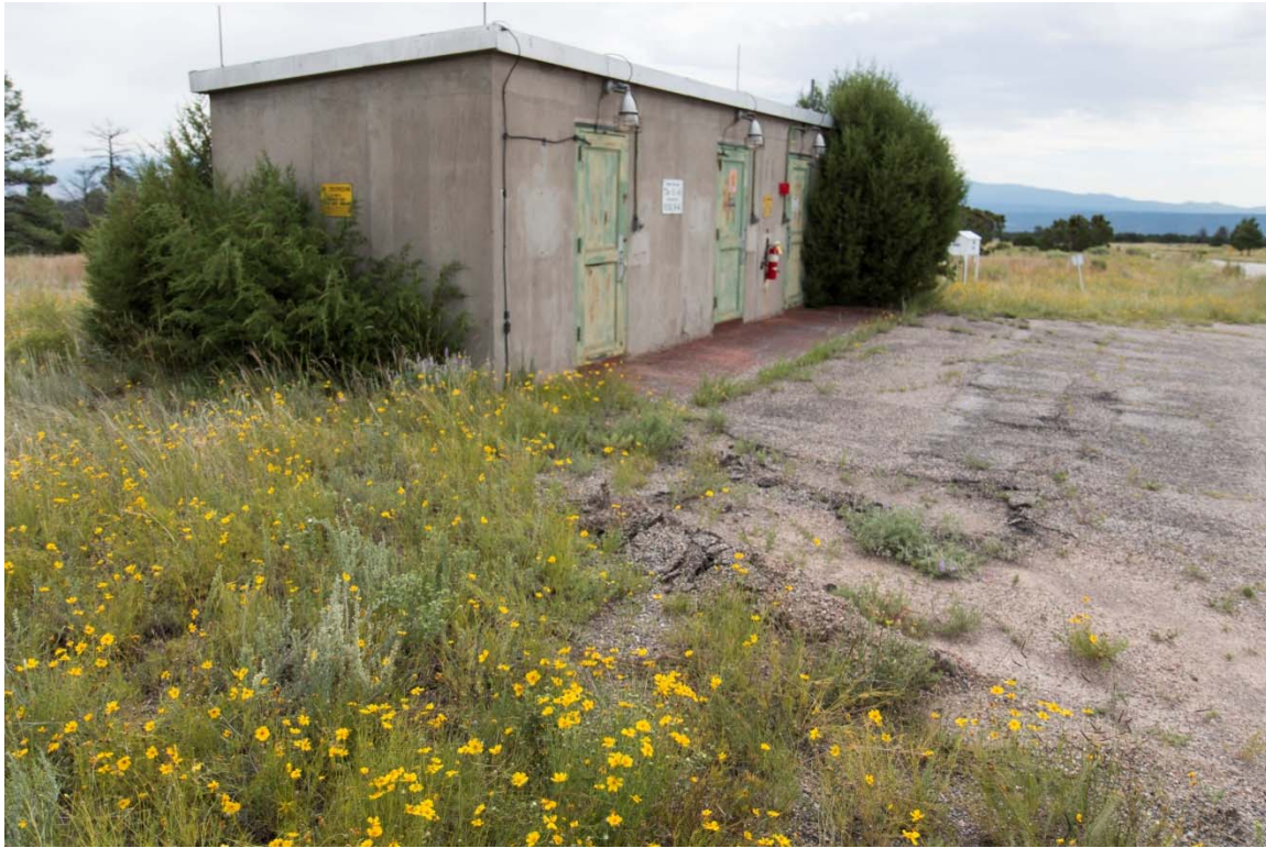
Figure I-3 Weathered asphalt on the south side of AOC 15-005(c), looking east
