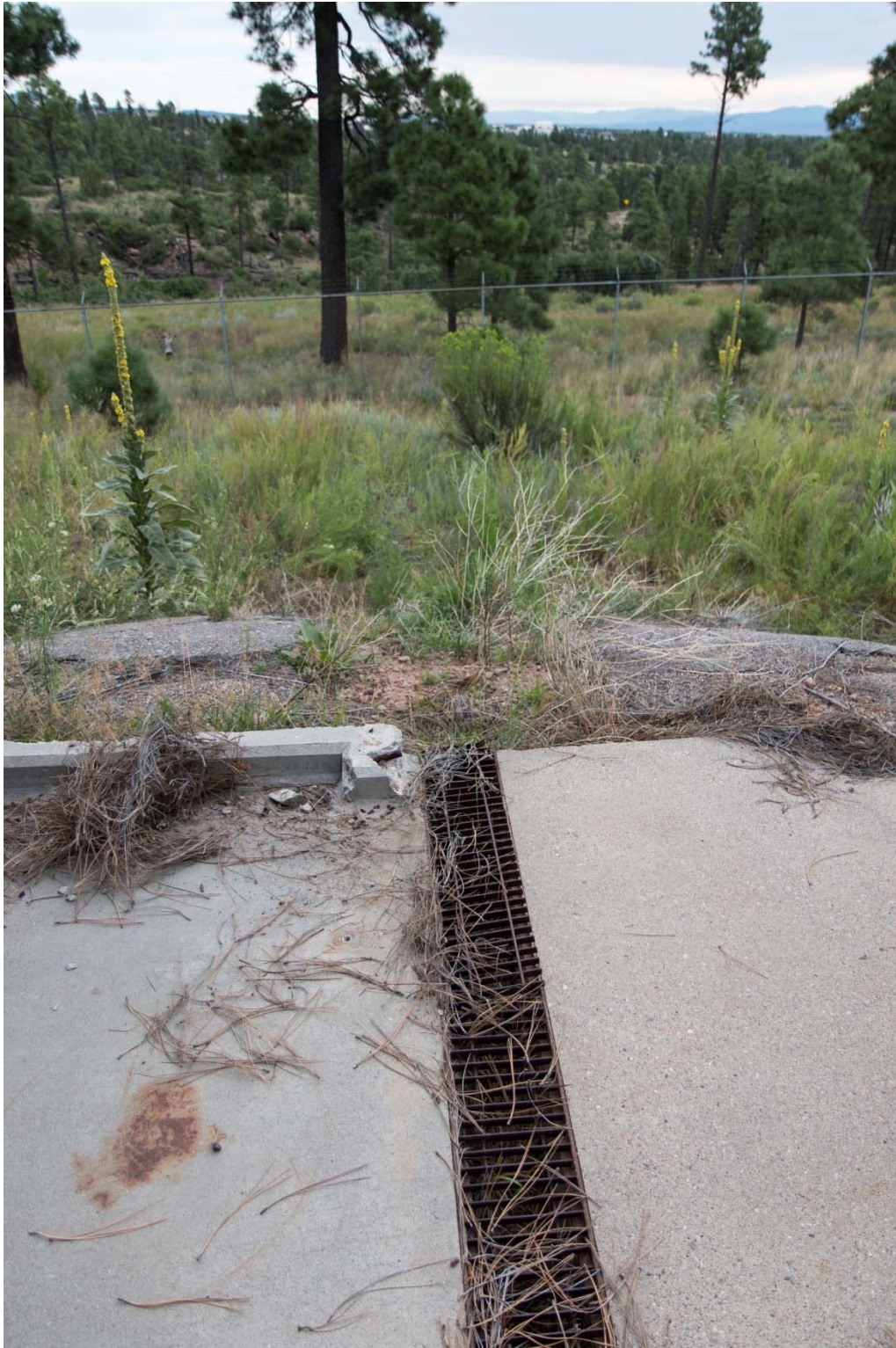
Figure I-12 Trench drain connected to eastern outfall at AOC 15-014(h) with asphalt debris, looking northeast
