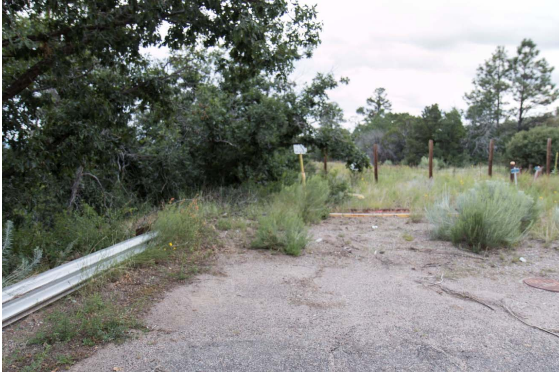
Figure I-17 Weathered asphalt area adjacent to SWMU 36-003(a) drainline and west of drain field, looking east
