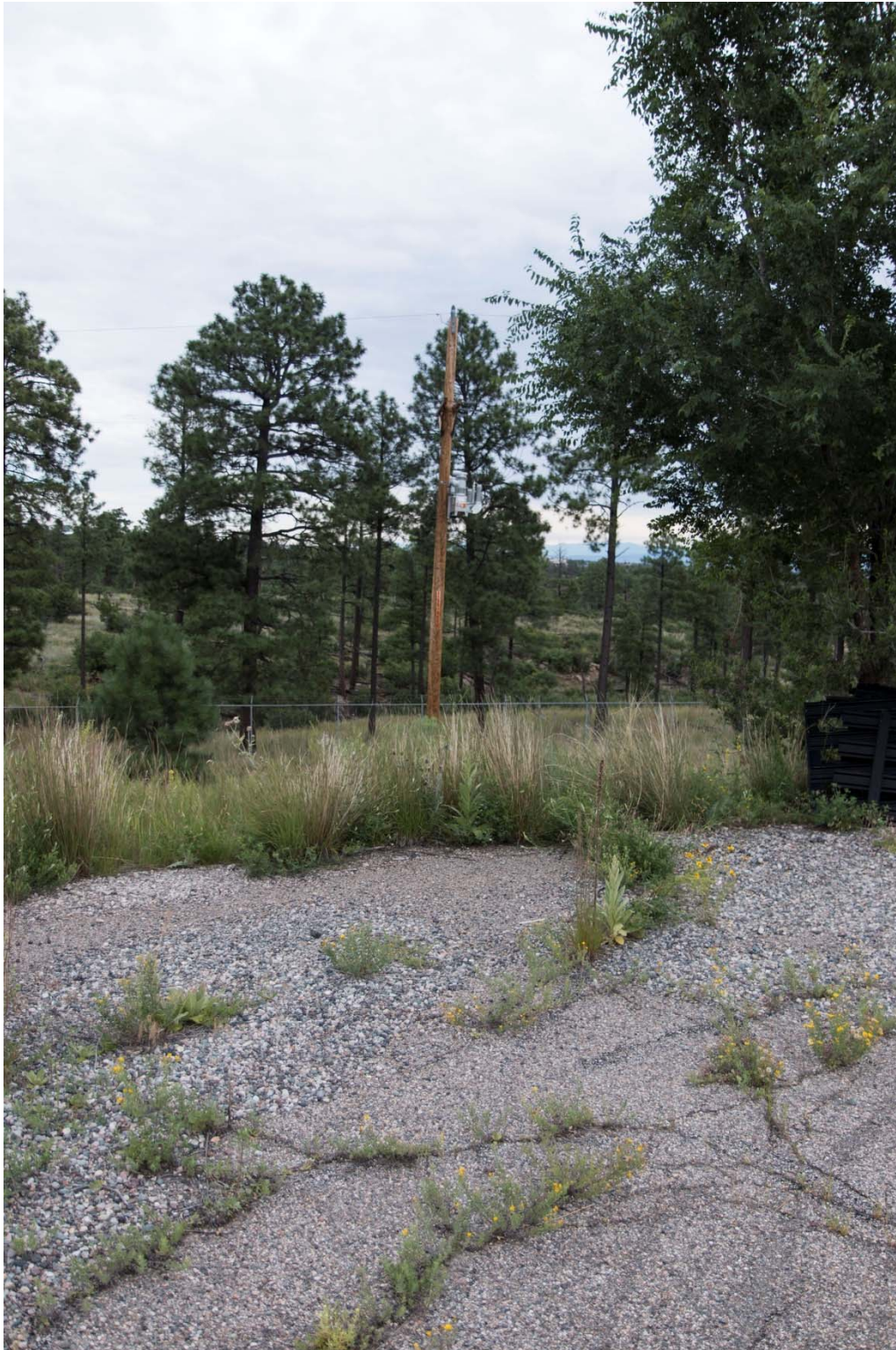
Figure I-15 Weathered asphalt pad above AOC 15-014(h) outfalls, looking northeast
