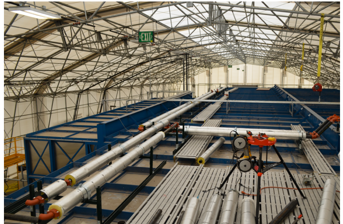
A supplemental cooling system was installed where the RNS drums are stored.
