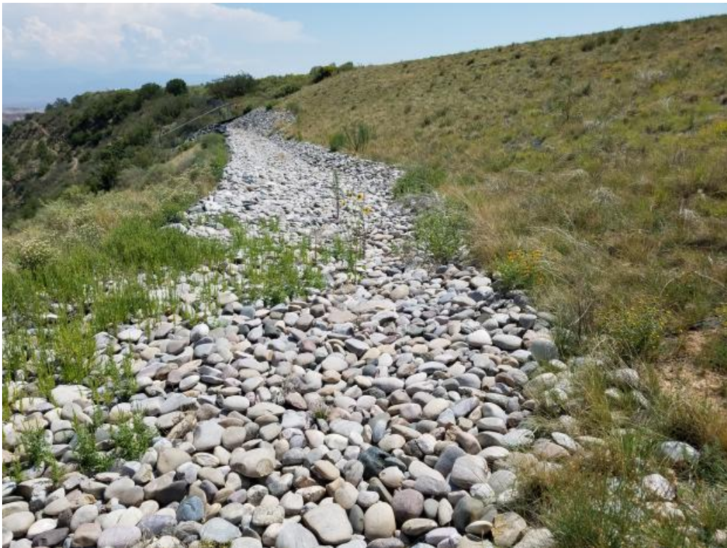
Picture 18. SE Berm - Adjacent to Airport Taxiway
