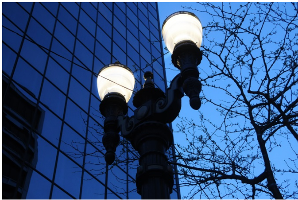
Figure 2. Ornamental post-top with LED retrofit
