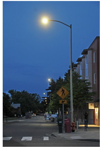
Figure 3. LED cobra head replacement luminaire
