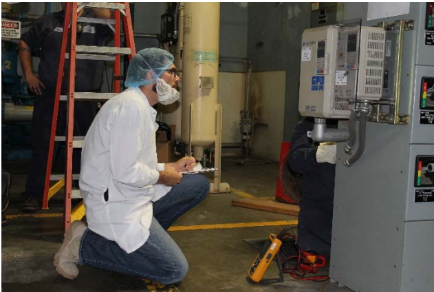
Keith Striby confirms proper placement of monitoring equipment and data loggers during a recent OSU IAC assessment.
