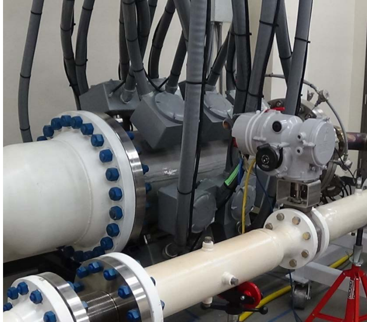
Figure 3-16. Primary Heater after Installation
