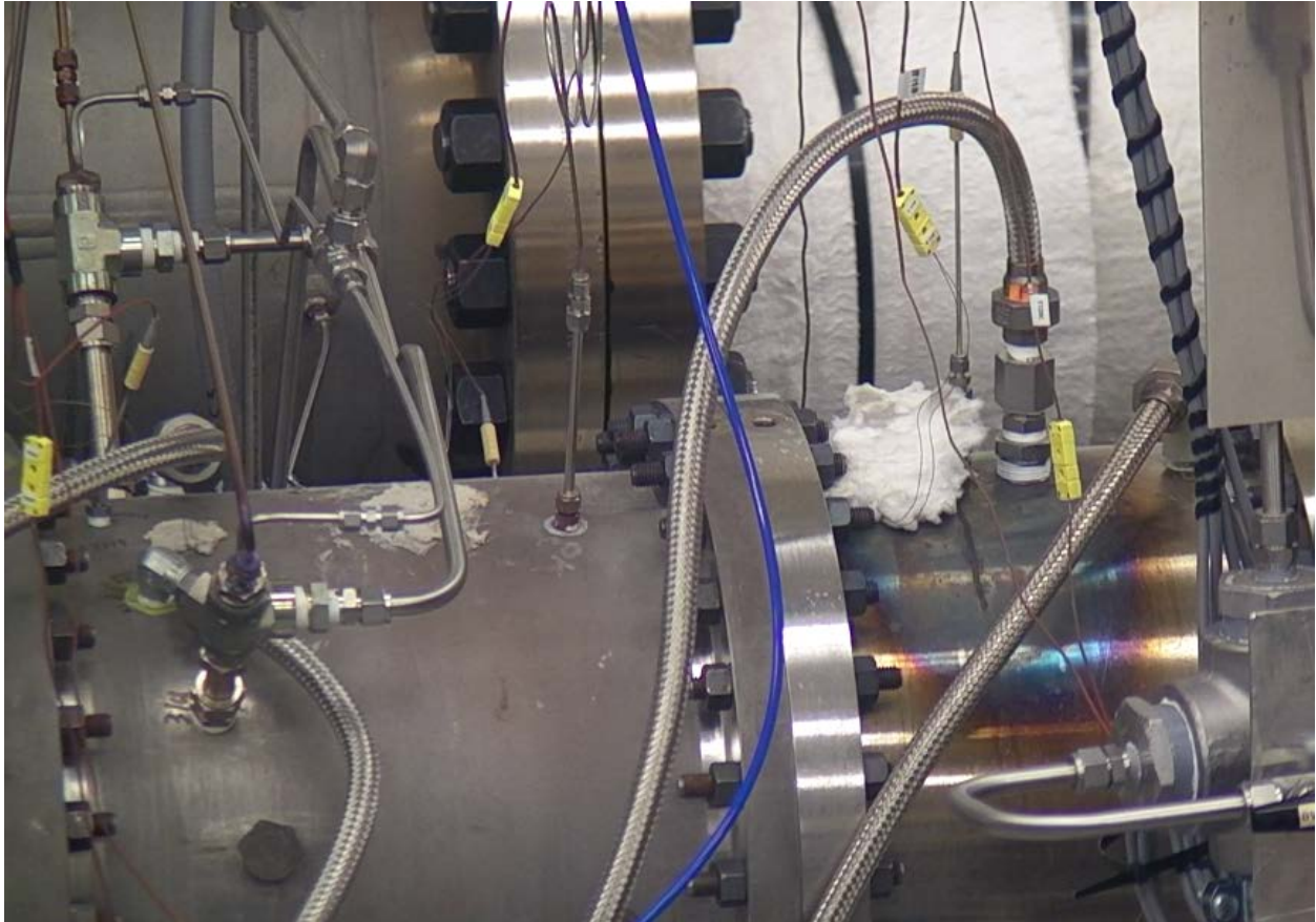
Figure 4-5. Combustor Housing with Moderate Discoloration
