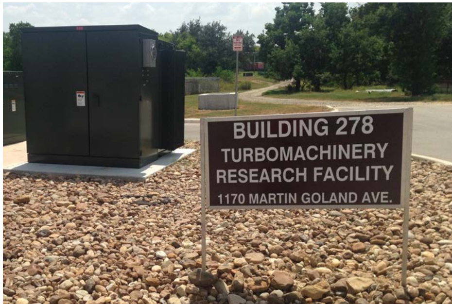
Figure 3-25. High-Voltage Step-Down Transformer
