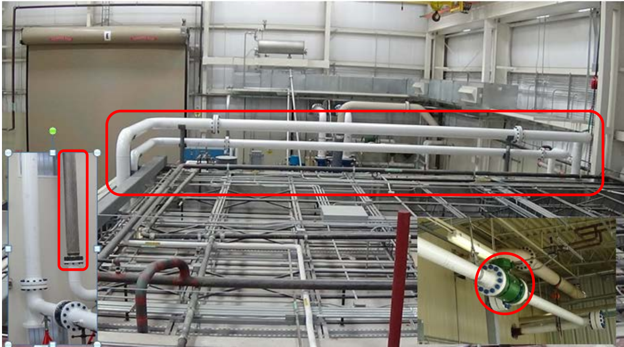
Figure 3-13. Combustor Facility Inlet and Exhaust Piping
