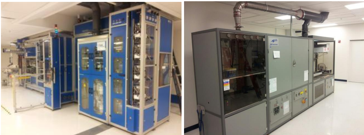
Figure 6: Production equipment installed at 6 Preston Court.
