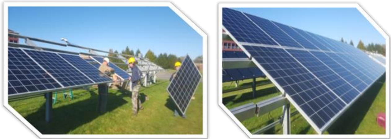
Figure 22: 50kW Installation of Direct Wafer modules at General Electric in Schenectady, NY
