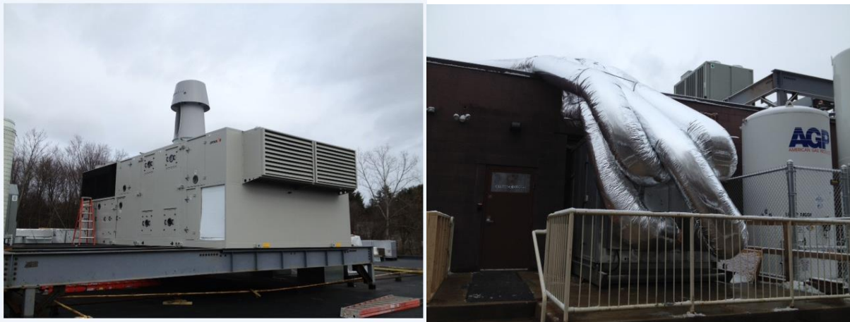
Figure 7: Energy Recovery Unit (left) from AnnexAir which did not meet specifications and temporary make up air system (right) installed to meet lab requirements.
