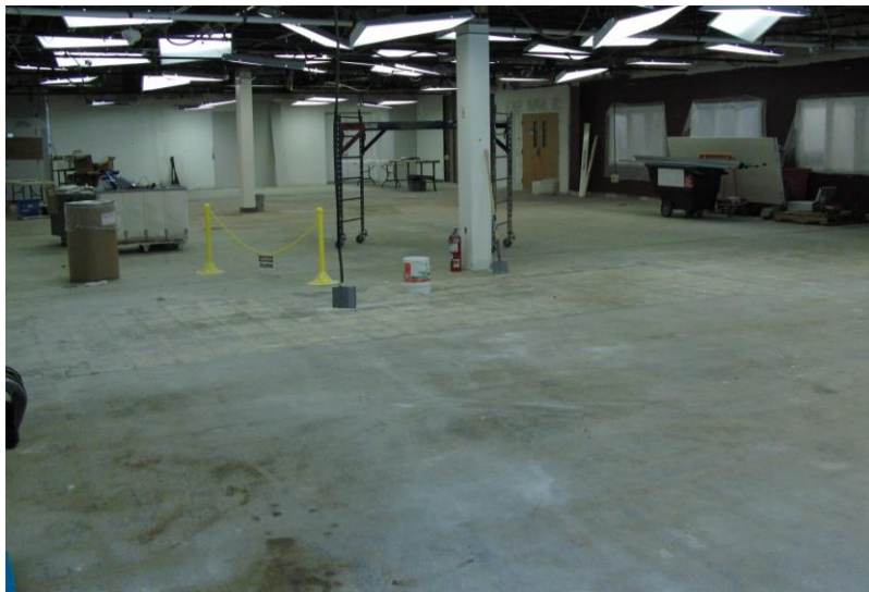
Figure 14: Empty Space for Expansion after Demolition as First Part of Phase 1b Construction.
