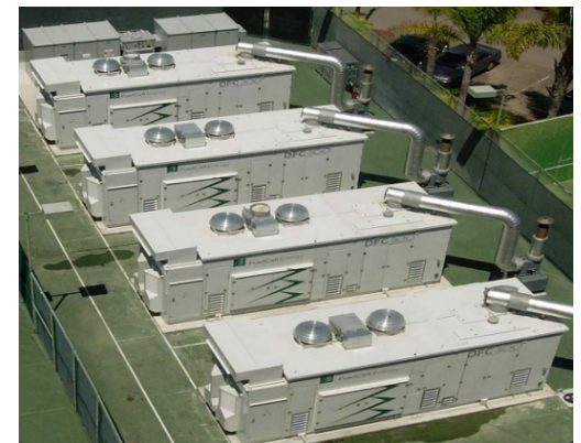
Hydrogen fuels stationary fuel cells provide primary power.
