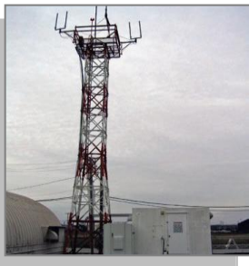
A 1-kW fuel cell system has been providing power for this FAA radio tower near Chicago for more than three years.
