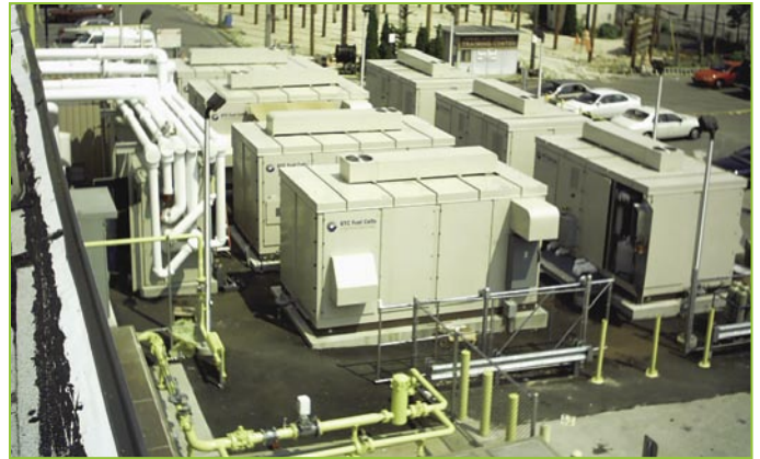
Figure 2. Seven 200-kW UTC fuel cells at Verizon’s central office of the future in Garden City, NY
