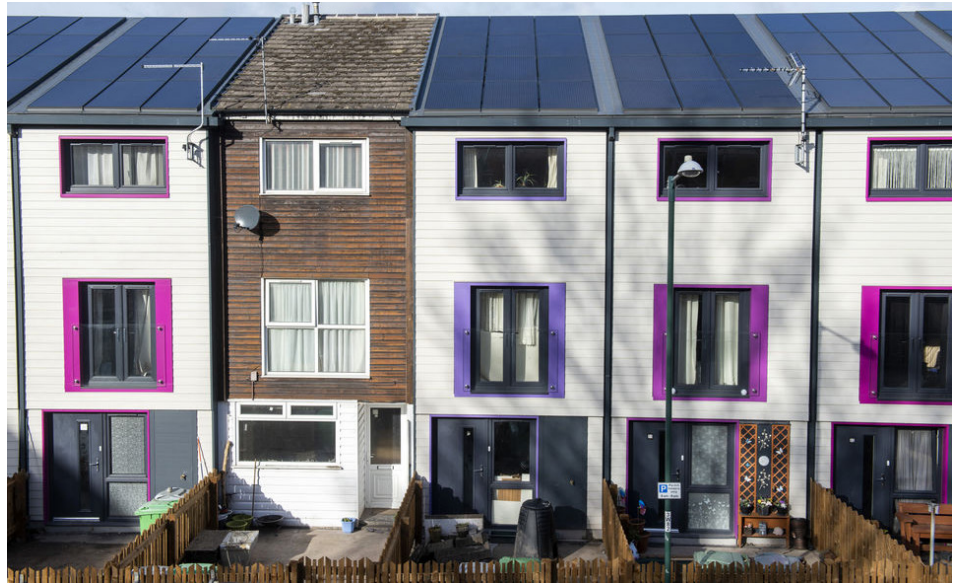
Zero energy retrofits can be completed quickly and without disruption to occupants by incorporating most of the improvements into the façade of the building. Photo credit Energiesprong.
