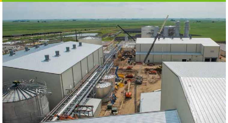
POET-DSM's Project LIBERTY cellulosic ethanol biorefinery in Emmetsburg, Iowa, was made possible with $100 million in BETO cost-shared funding. Photo courtesy POET-DSM.
