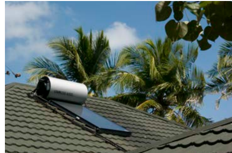
A rooftop solar water heating program in Barbados met with success thanks to effective financial incentives and government support. Photo from iStock 6923507
