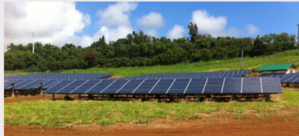
Analysis indicating high penetration of variable renewable generation would not compromise grid stability or power quality helped de-risk the installation of this 1.2-MW PV array on Kauai. Photo by Jamie L. Keller, NREL 21774
