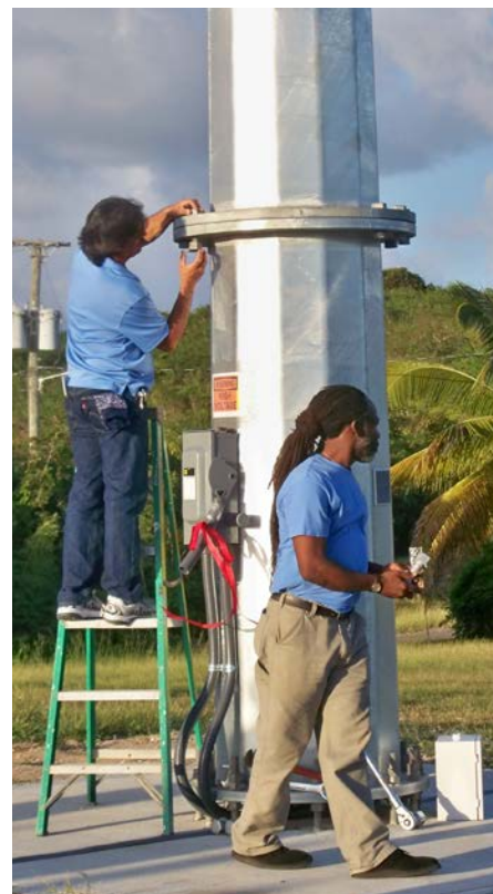
Workers install a 10-kilowatt wind turbine at the St. Croix Reformed Church and Kindshill School in St. Croix, U.S. Virgin Islands. Photo from Don Buchanan, Virgin Islands Energy Office, NREL 20418
