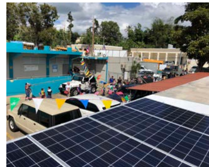
Solar panels on the roof of one of 10 Puerto Rico schools where solar and storage microgrids were installed to power critical loads. Photo from RMI
