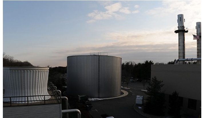
Princeton University's sophisticated control systems enable it to maximize the financial benefit from its CHP system based on varying prices on the energy markets. Photo credit: Princeton University
