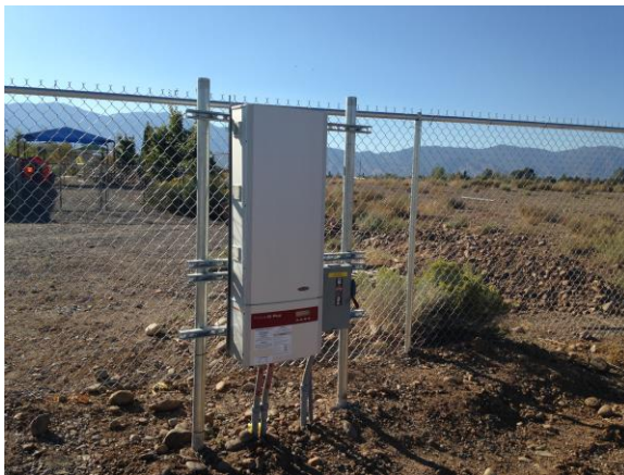
Installed inverter and electrical components
