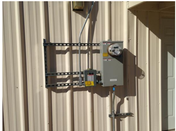
Installed solar meter and junction box
