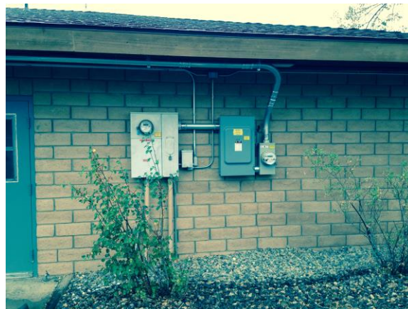
Installed solar meter and junction box
