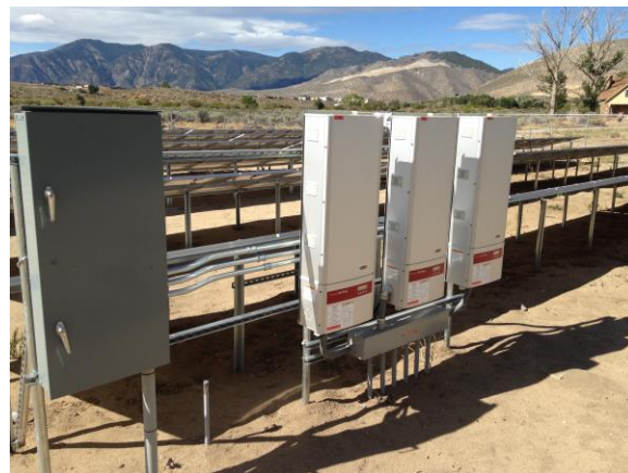
Installed inverter box and electrical components
