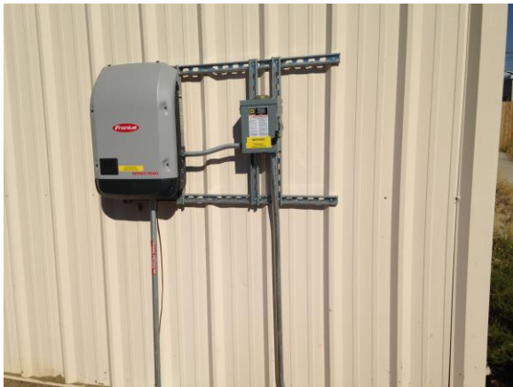
Installed inverter and electrical components
