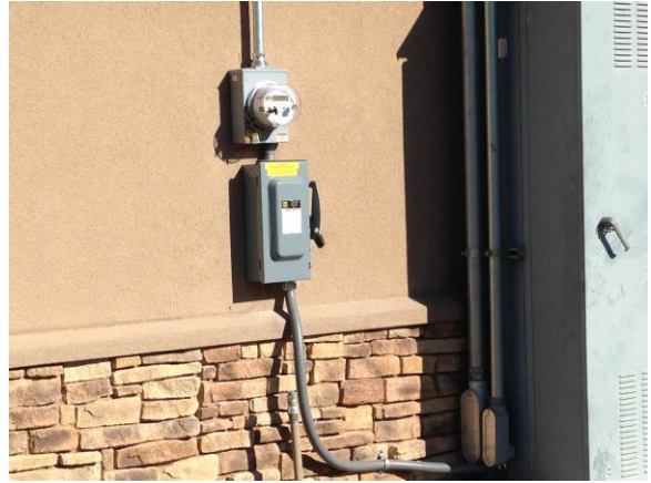
Installed solar meter and junction box
