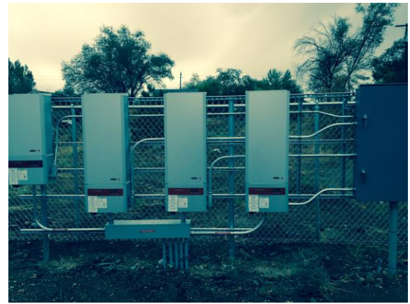
Installed inverter and electrical components
