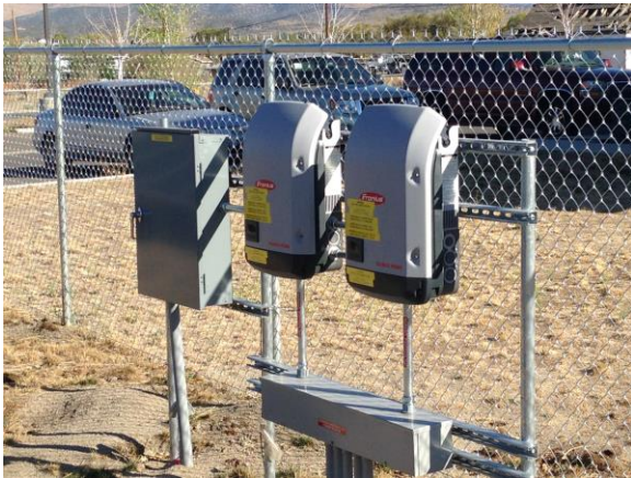
Installed inverter and electrical components
