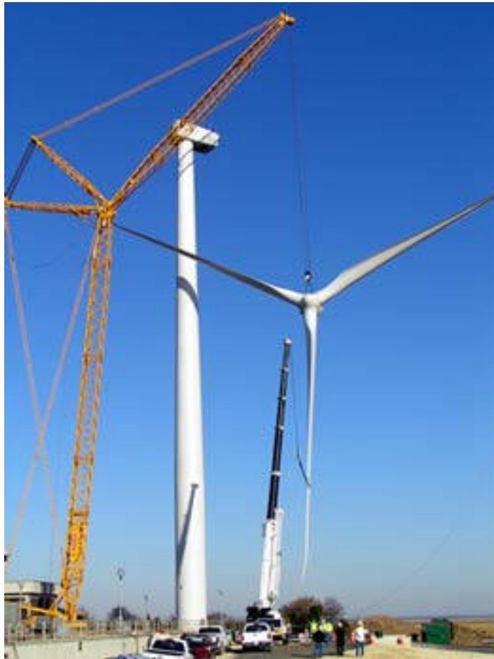
Figure 5. Example illustration of 1.5 MW wind turbine assembly, on an 80 m (260 ft) tower, in Atlantic City, NJ.
