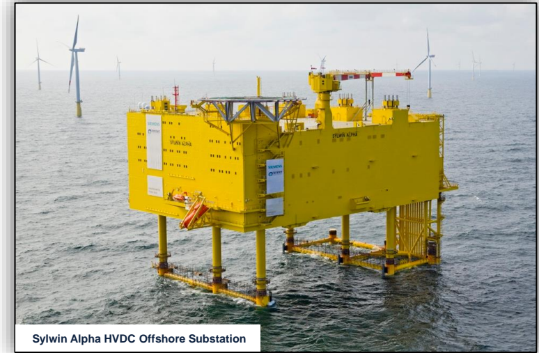
HVDC Converter Substation
