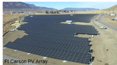
Fort Carson PV Array
