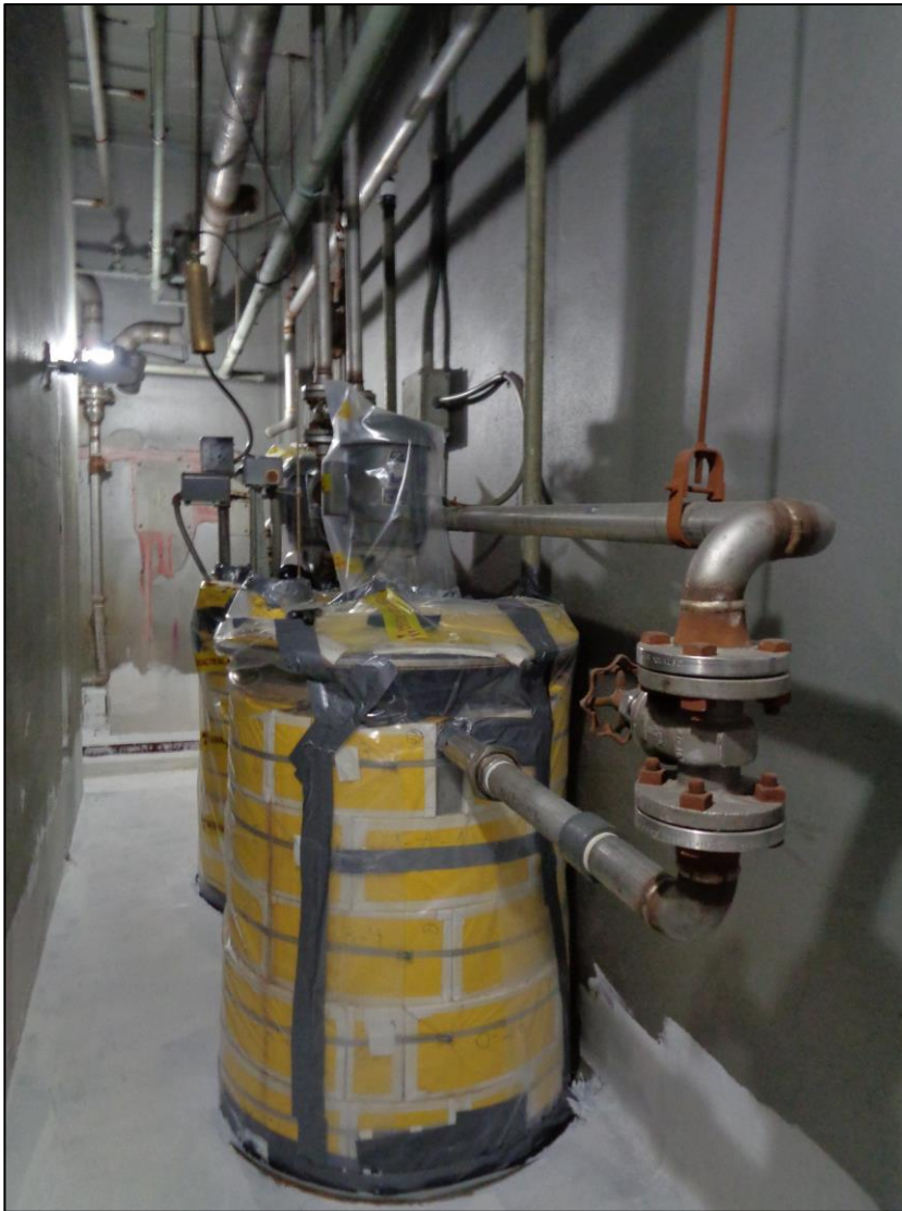
Figure 34. E1 Interceptors as-left condition. View from west
