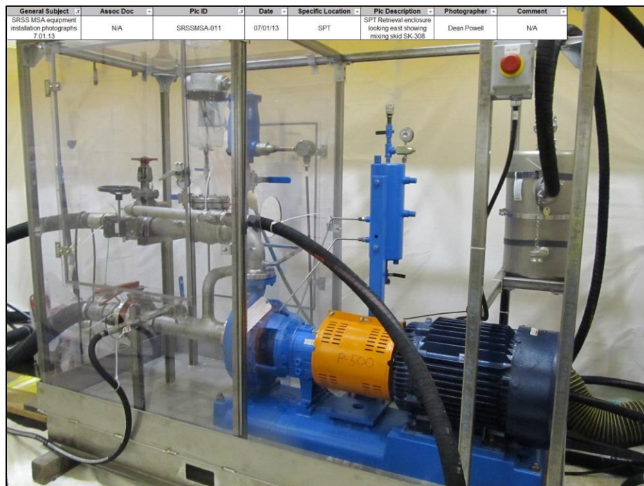
Figure 13. Mixing skid for the Sludge Retrieval and Solidification System
