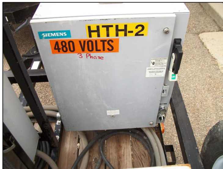
Figure 4. Typical Disconnect Switch
