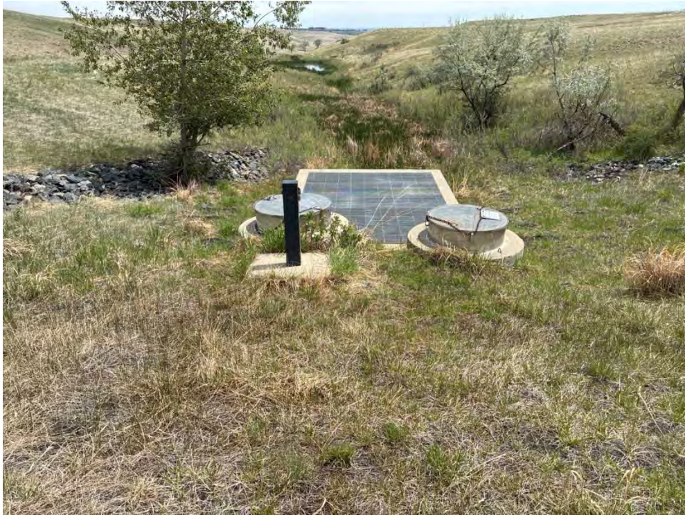
Figure 7. Looking East-Northeast at the Present Landfill Treatment System, Which Was Functioning Properly. Small amounts of bio-growth were removed from the North and South Manhole Outlet Pipes, treatment unit outlet pipe, and system outfall using a mechanical pipe cleaner as part of routine preventative maintenance.
