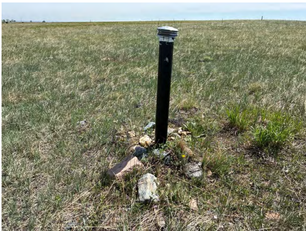
Figure 6. Looking East-Northeast at a Barometric Gas Vent on the Present Landfill Cover, Which Were all in Good Condition
