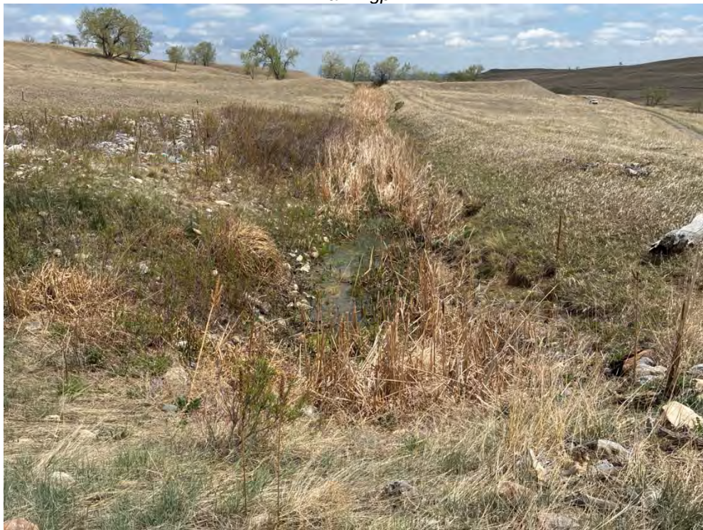
Figure 13. View Looking East at the SID, Which Receives Groundwater from the ESSD Outfall and an Interceptor Drain on the Eastern Hillside and Had a Flow Rate of Approximately 1–2 gpm.
