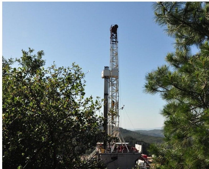
Drilling for steam at Bottle Rock in California. Photo credit: Betsy Phillips, via the Geothermal Rising photo contest
