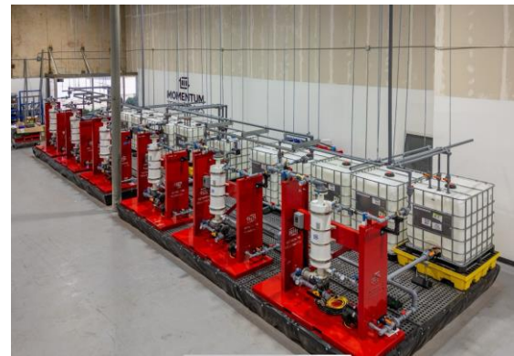
MSX Facility at Momentum Technologies
